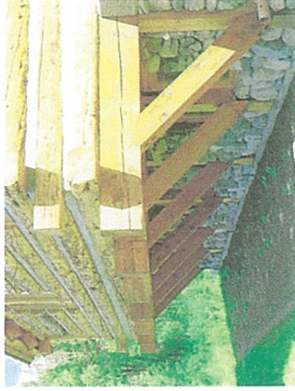
▲ Cantilever supported with timber bracing.
